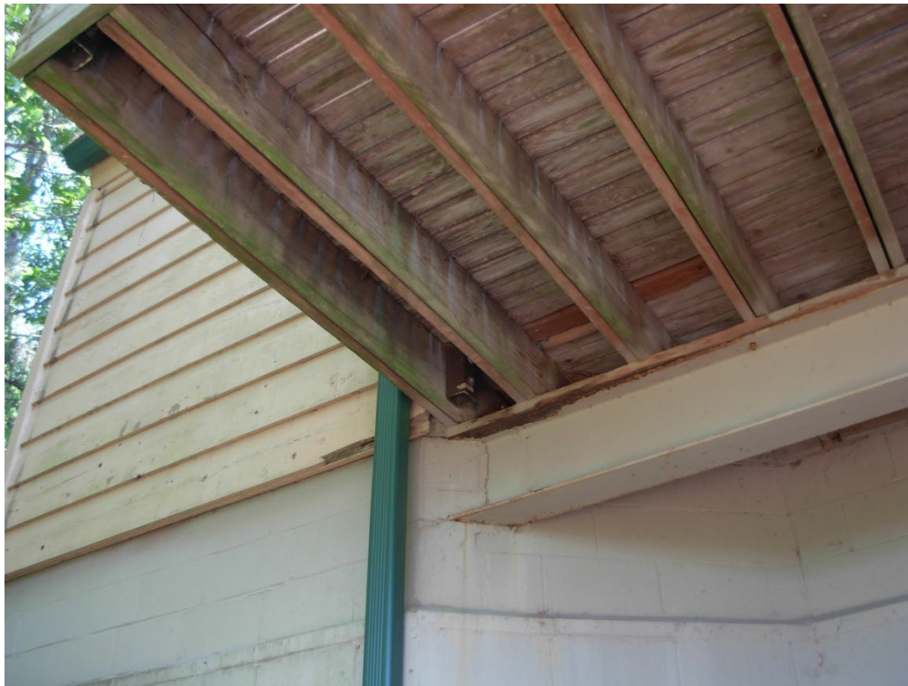
Photo 20: The steel beam bearing at the Northeast corner of the deck looks better.
