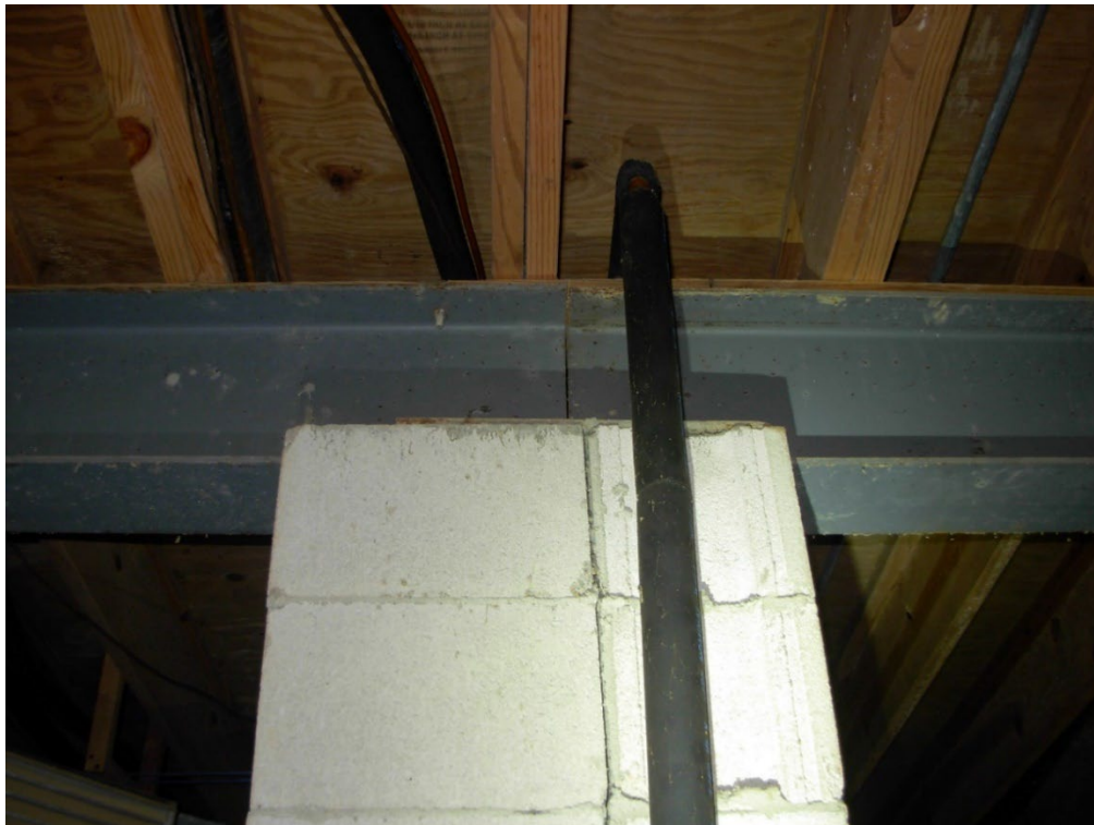
Photo 28: The floor girders in the crawl-space are steel beams bearing on concrete block piers. This condition is structurally acceptable and appears to be in good condition.
