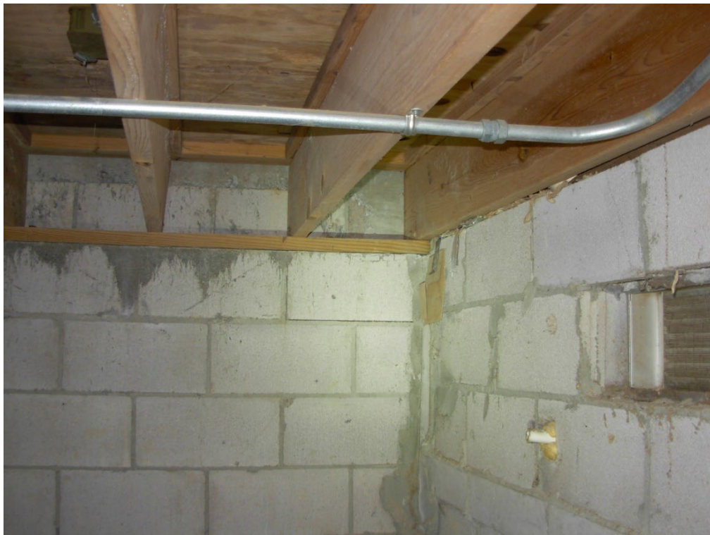
Photo 25: The concrete block foundation wall inside the crawl-space appears to be in acceptable condition, despite several mortar joint cracks.
