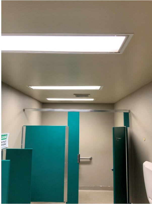
Photo 40: Existing fluorescent recessed lighting in restroom.
