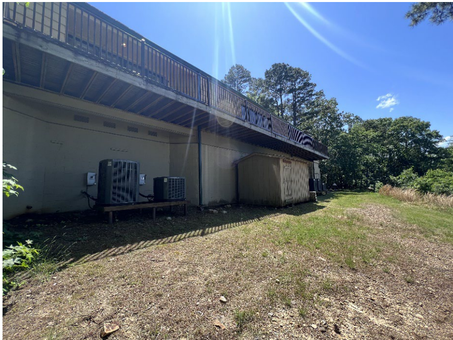
Photo 37: Existing Condensing Units
