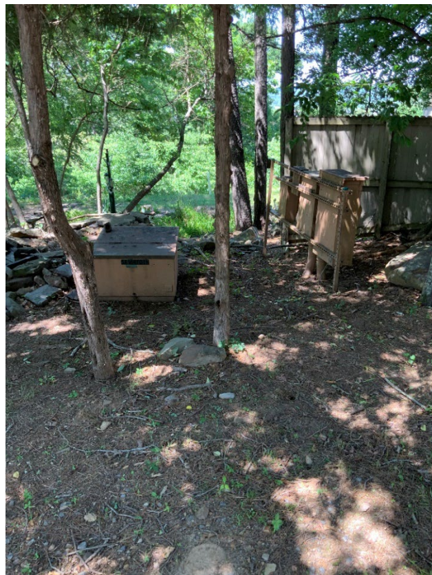
Photo 45: Existing utility transformer and service disconnect.
