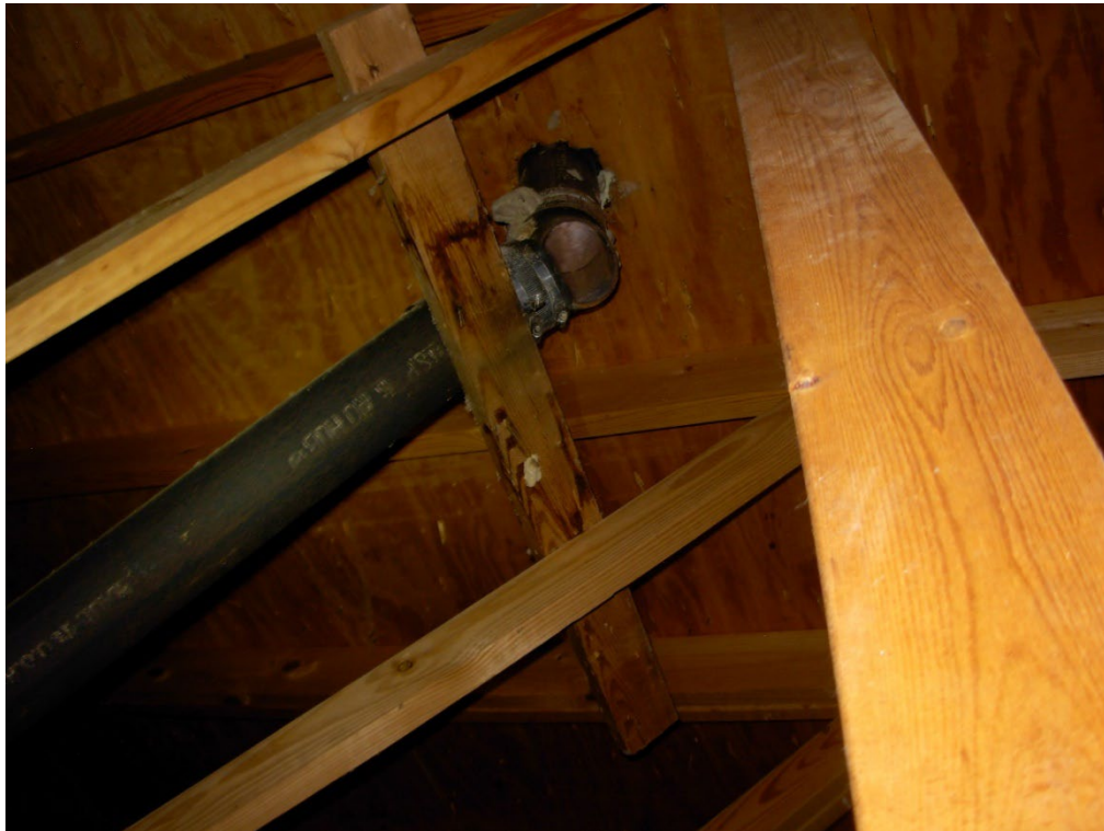
Photo 9: In the Meeting Room near the south wall, there is a vent stack that is disconnected and needs to be reattached.
