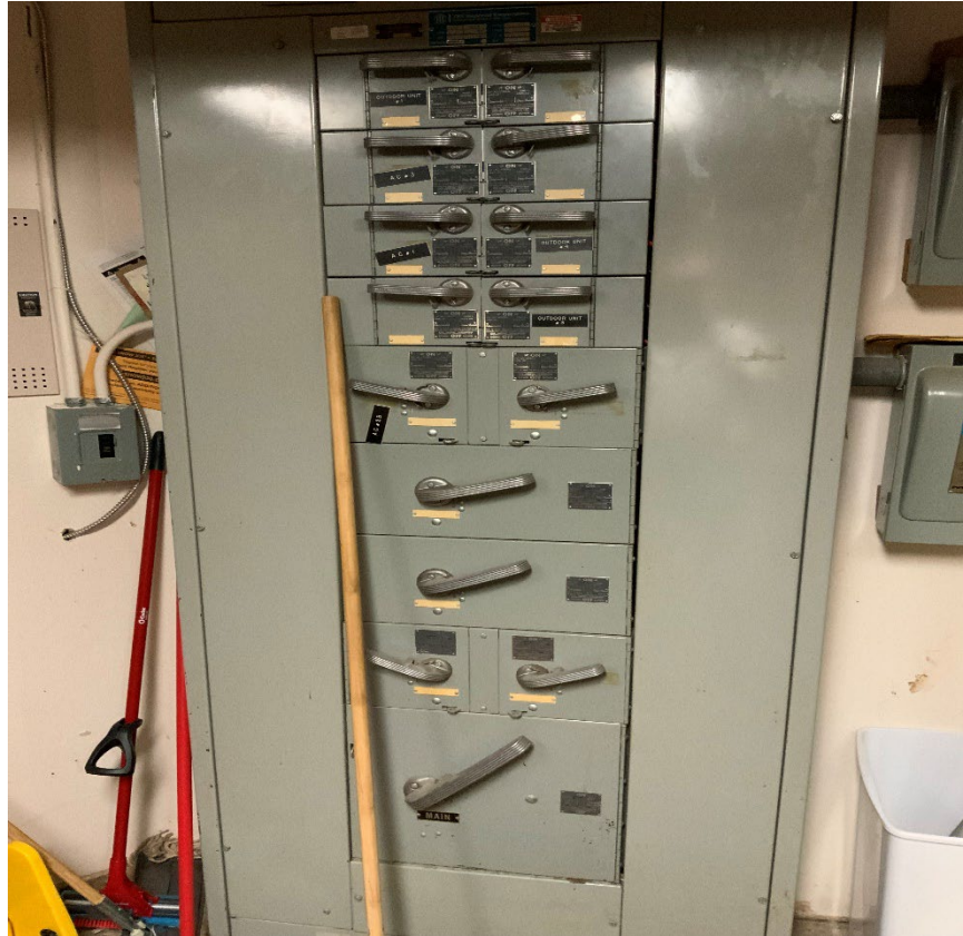
Photo 38: Existing MPD 400A 240/120, 3 phase, 4-wire.
