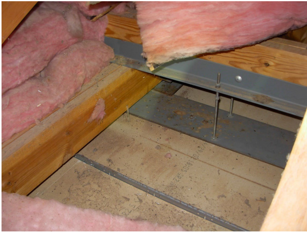
Photo 8: The existing operable partitions are supported by steel tracks and stiff-backs that are supported by the wood truss bottom chords. The 2x4 acoustical ceiling tile ceiling is within a few inches of the bottom of the trusses.
