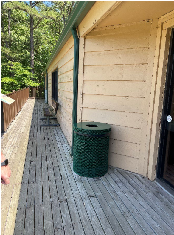
Photo 16: Deck. Accessible from Exhibit Area and Meeting Room. Window from Discovery Room. Structural images to follow. Deck is approximately 6' wide x 74' in length.
