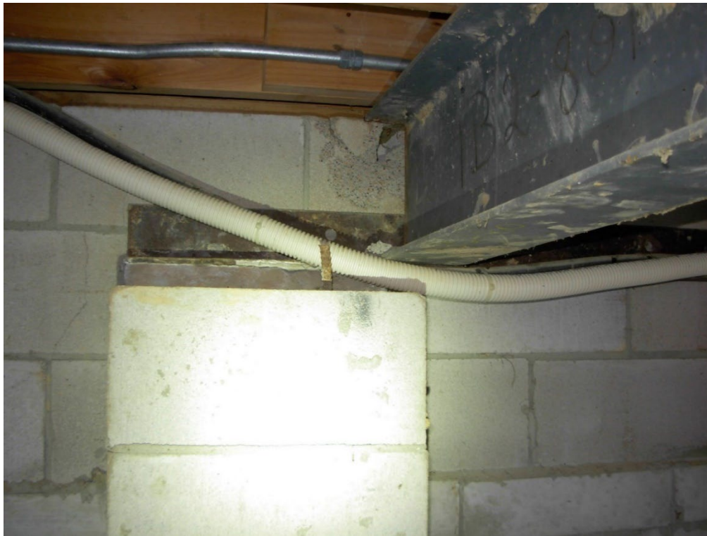
Photo 30: Close-up view of the steel girder bearing on the steel angle. The angle is bolted to the concrete block wall and bears on a grout bed on the pilaster.
