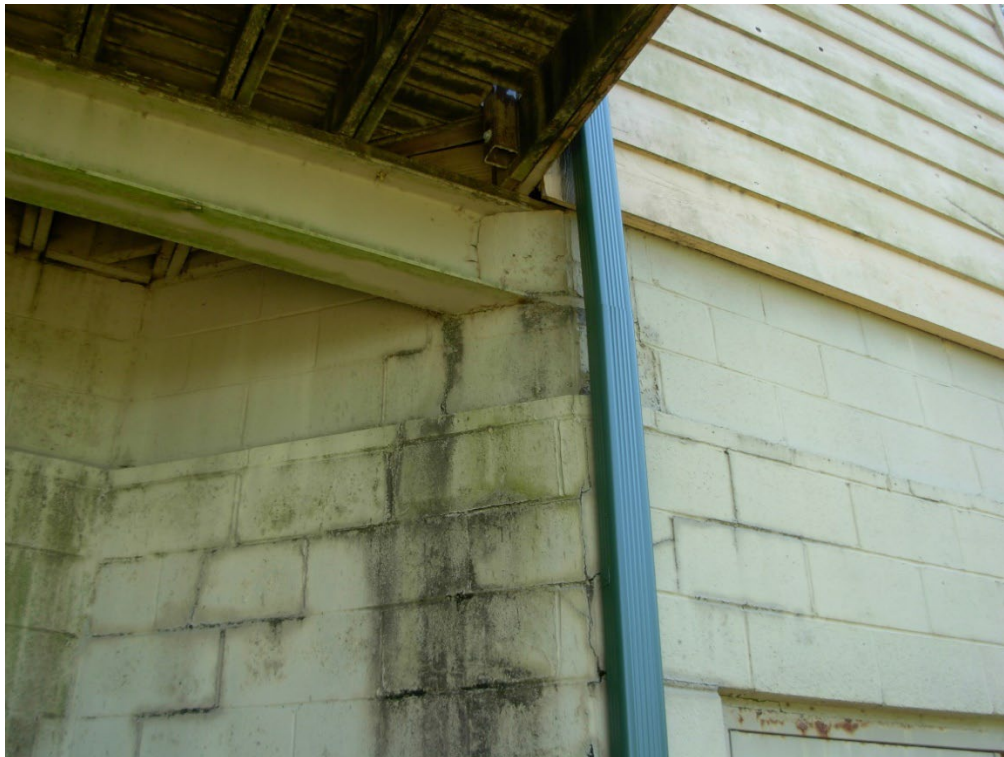
Photo 18: There are cracks and water streaking below the Northwest corner of the deck. There is a steel beam bearing on the concrete block that is adding some thermal expansion and contraction forces to the wall. This will need some attention if the deck is replaced or retrofit.
