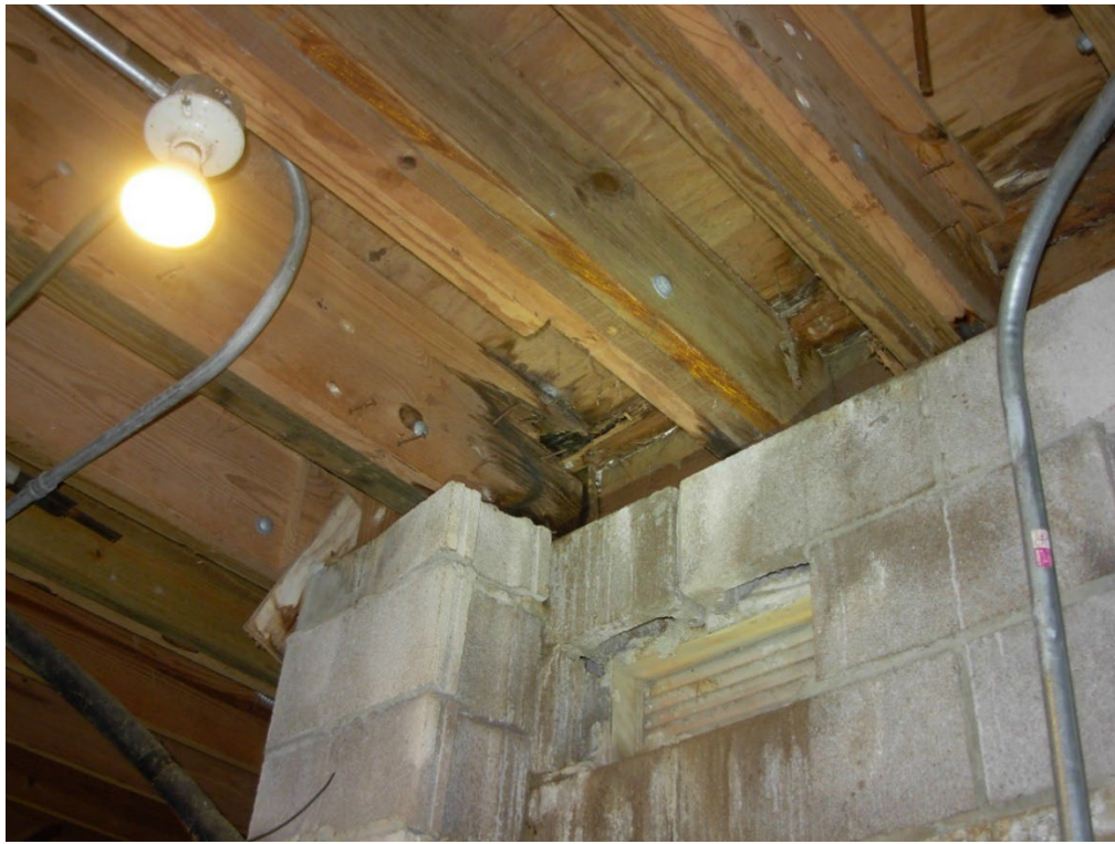
Photo 32: Water damage to the wood decking and floor joists at the back wall below the deck. This area has enough structural damage to be of concern of causing load support issues for the deck and back wall of the building and needs to be addressed ASAP.
