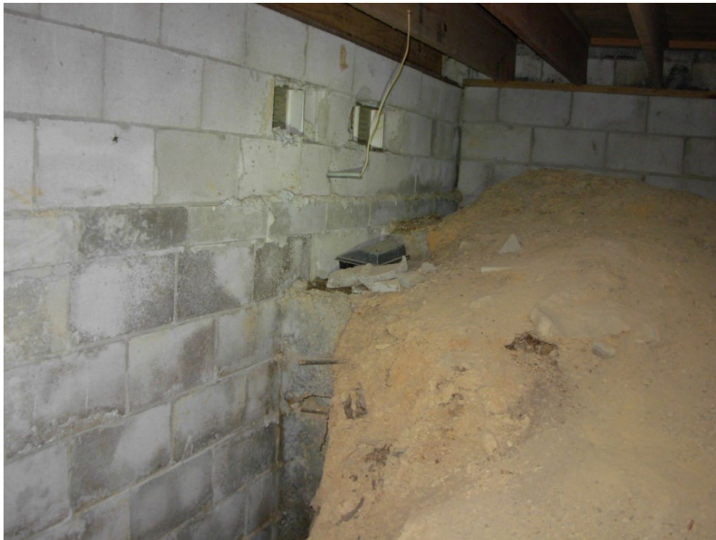
Photo 27: The East side foundation wall is in good condition. It has a large footing step that is exposed, but this too looks okay.
