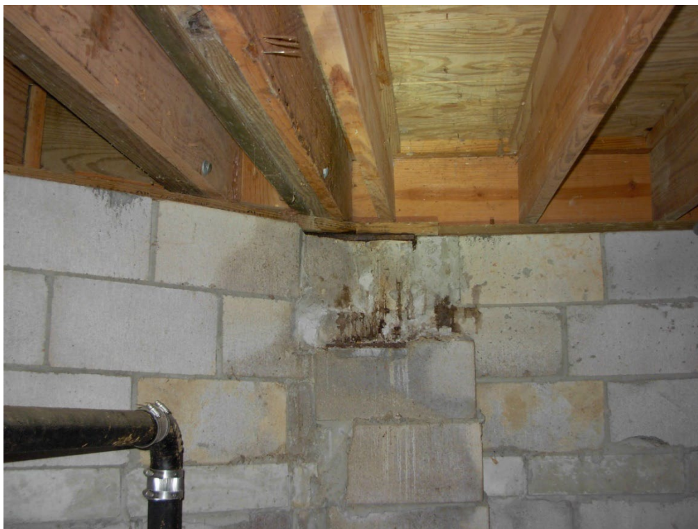
Photo 21: Overview of the steel beam bearing from inside the crawl-space. This condition looks rough, but structurally it is acceptable.
