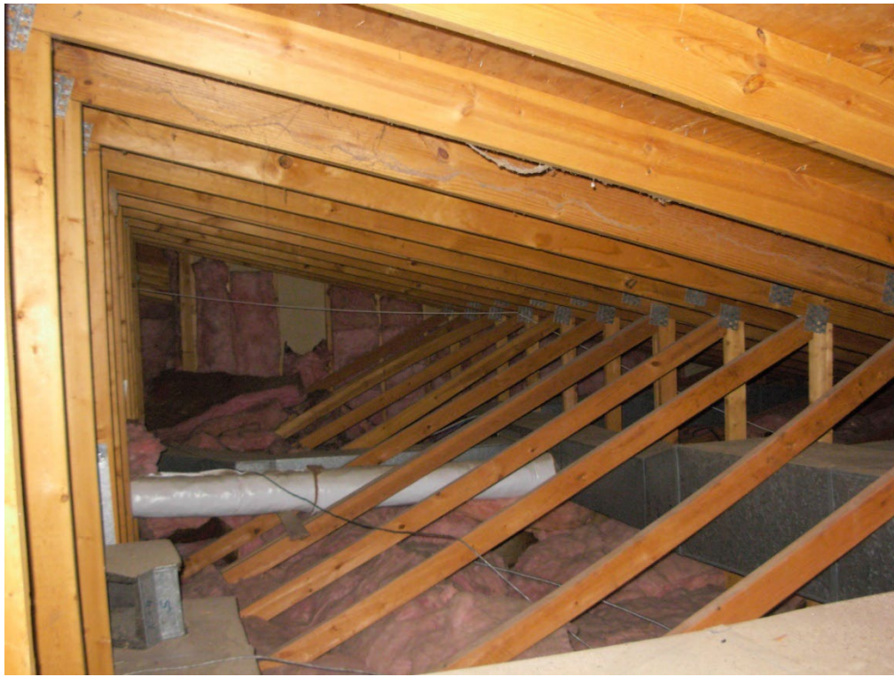
Photo 6: The attic space above the meeting room is wood trusses with the bottom chord just above the ceiling.
