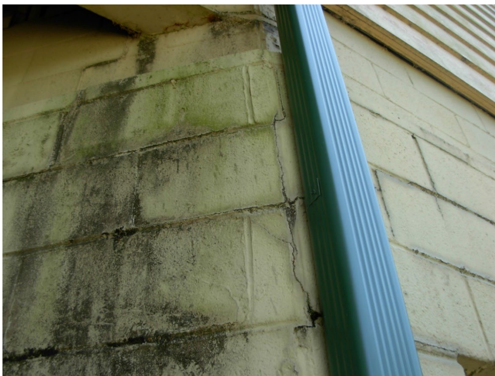
Photo 19: Close-up view of Northwest corner beam bearing. This looks worse than it is due to the water issues. The beam bearing and concrete block cracks are not in danger of failure.
