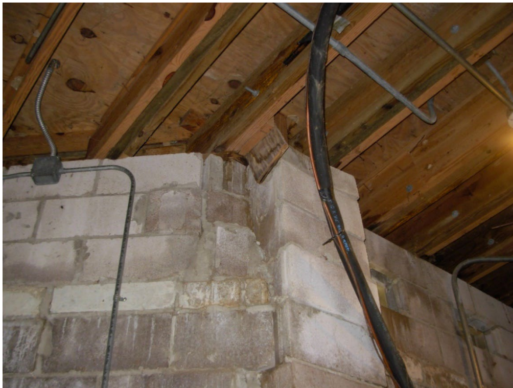
Photo 31: There is water damage to the wood decking along the back wall below the deck. If the deck is replaced, these areas need to be remediated with new wood and new flashing & waterproofing.
