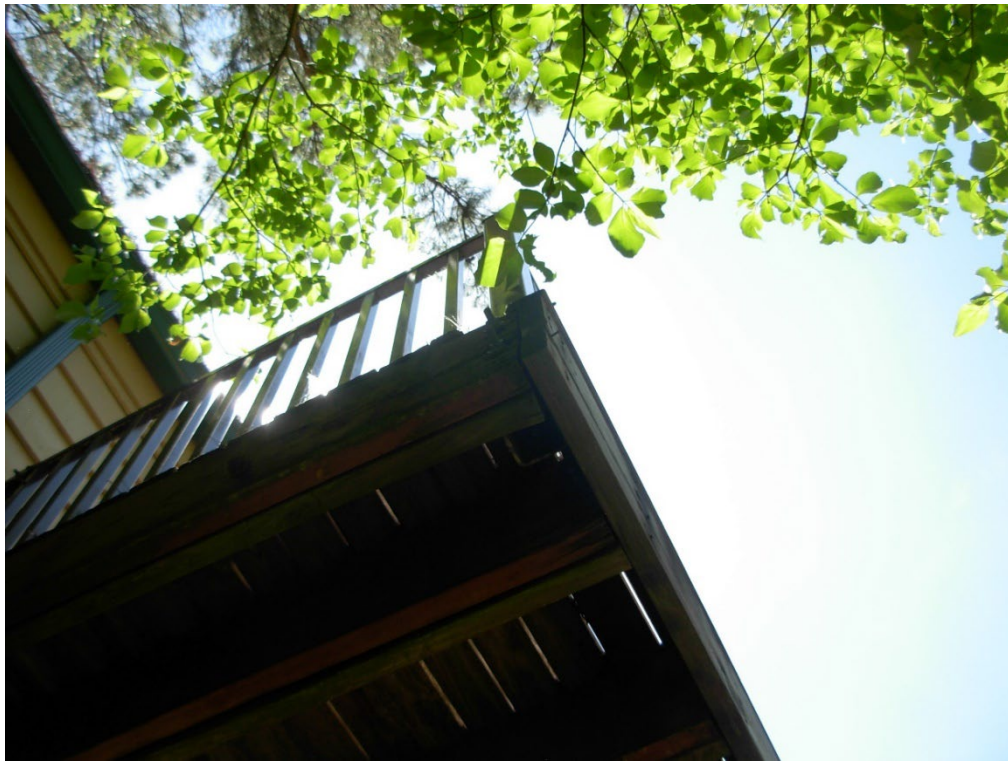
Photo 24: The Northeast outside corner of the back deck has some separation of the wood members, due to weathering and warping of the wood. This wood separation can decrease the load capacity and safety of the guardrail system.
