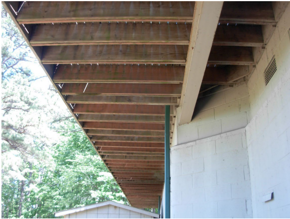
Photo 22: The back deck is cantilevered to the north and showing signs of age and weathering.
