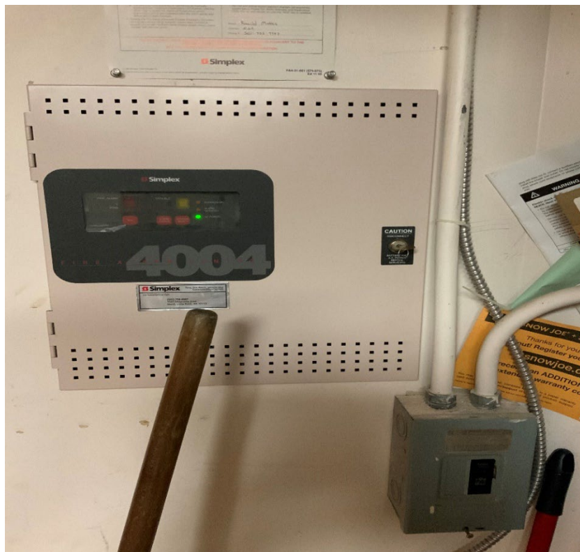
Photo 39: Existing fire alarm system.
