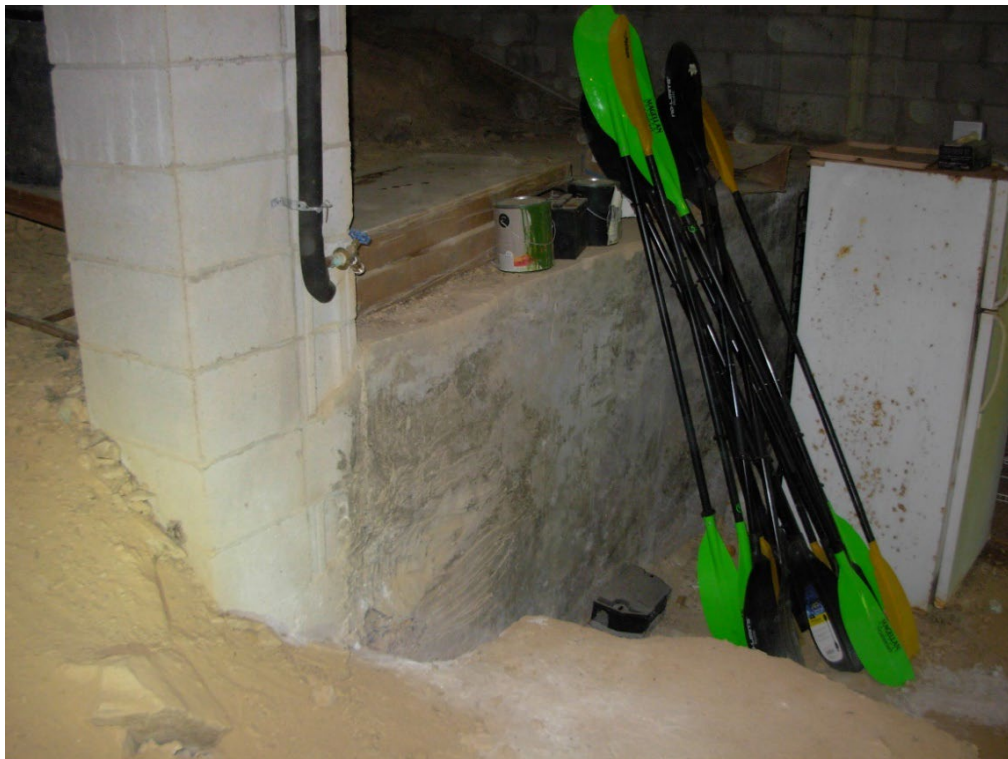
Photo 33: There is a concrete wall in the crawl-space that allows for a concrete pad in the Northwest corner. This wall is in good condition. The full length of the crawl-space could be similarly excavated and walled off to allow for more useable space, as desired.
