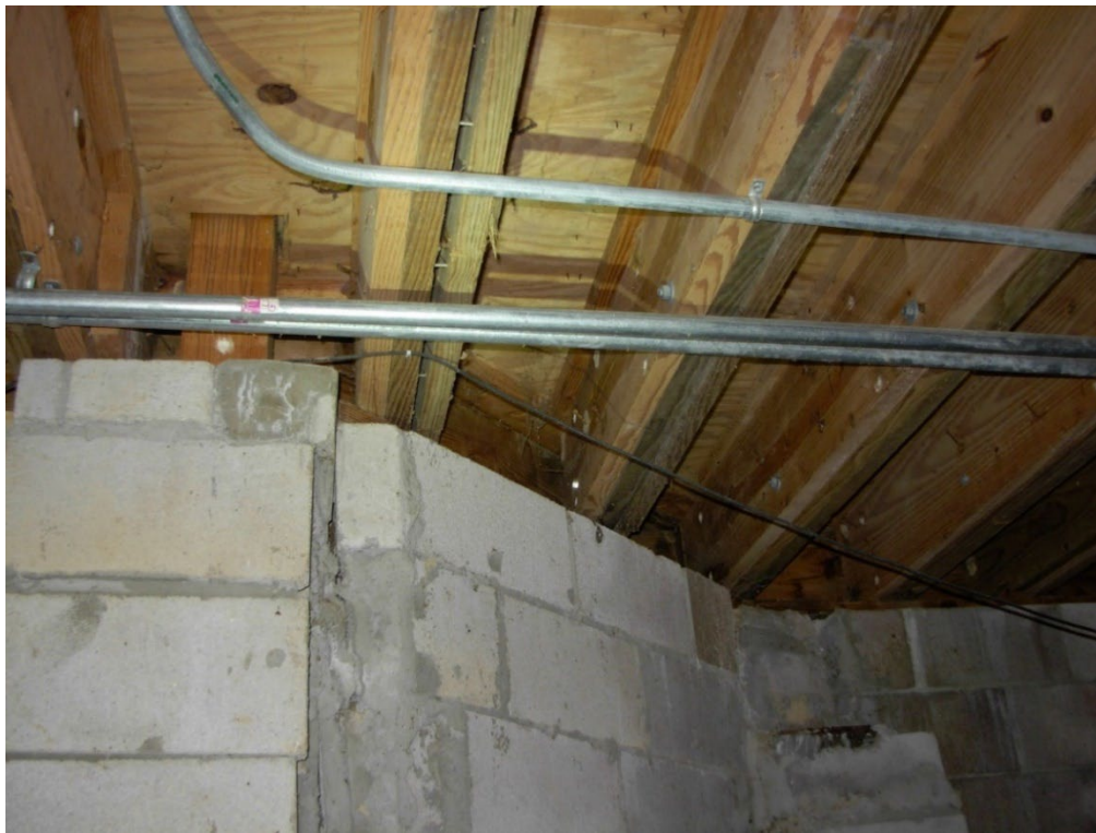
Photo 26: Crawl-space view of the back deck cantilever joists lap spliced to the floor joists. Some visible separation has occurred, but most of the members are in good shape. However, the deck likely needs to be replaced soon. I recommend cutting of the cantilevered joists and placing new exterior columns and beams at the outside edge of a new deck. This will allow the deck to be enlarged and have a higher load capacity.
