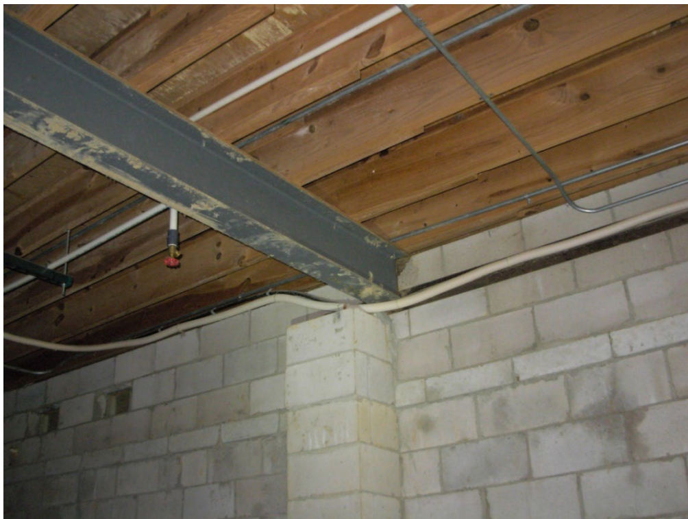
Photo 29: On the west end of the steel girder, the concrete block pilaster was apparently misplaced, so a steel angle was added to support the beam. This condition is not ideal but appears to be working.
