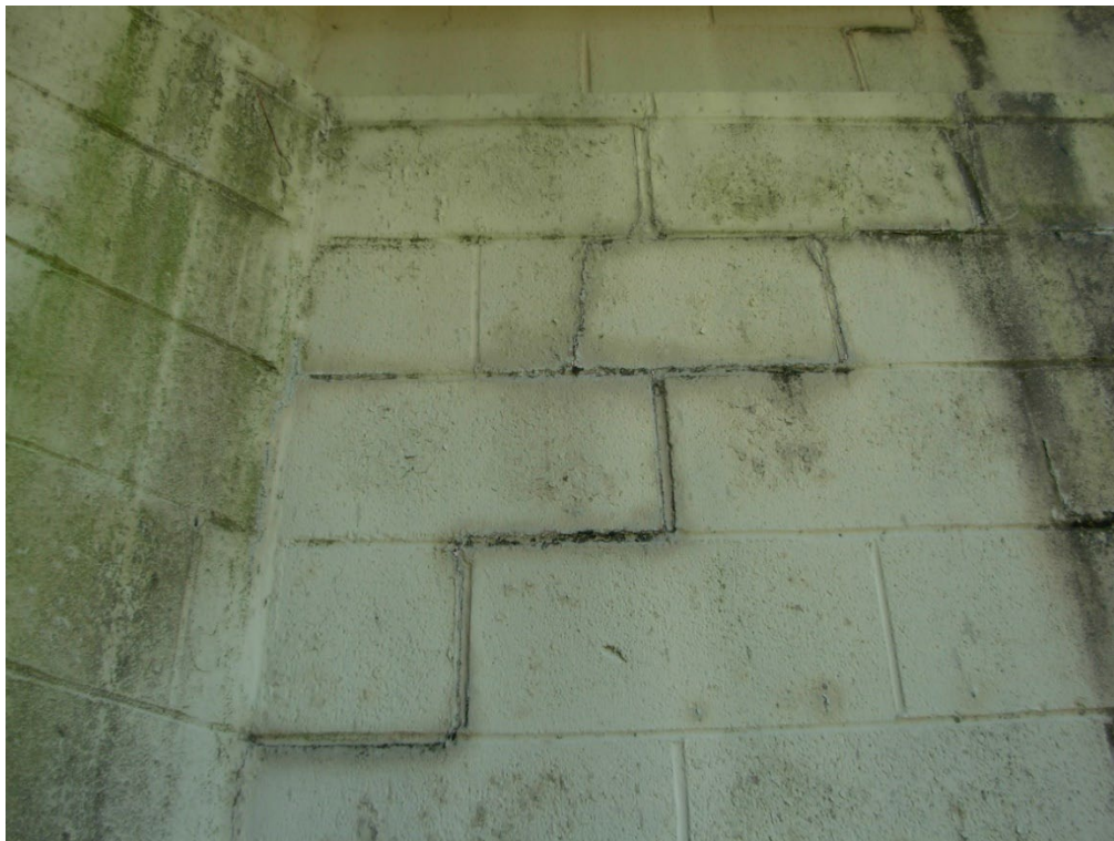
Photo 17: There are a couple of cracks in the concrete block stem wall in the Northwest corner. It appears there was some settlement shortly after the building was constructed, as these cracks were documented in 1992 and appear to be basically unchanged. I do not see these as a structural issue, unless the loading conditions of the walls are changed by any future improvements or adverse events.
