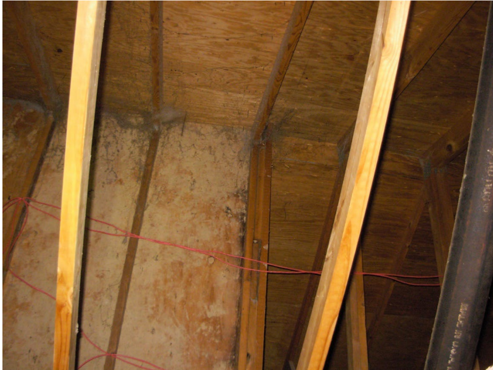
Photo 7: The end and front entry clerestory walls are built into the truss profiles.
